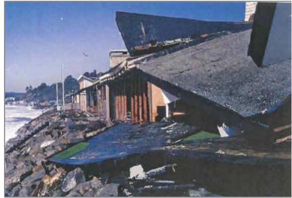
Figure 5-2: Damaged homes near Seacliff State Beach and Rio Del Mar during the 1982-83 El Niño. Source: Photo courtesy of Gary Griggs.
